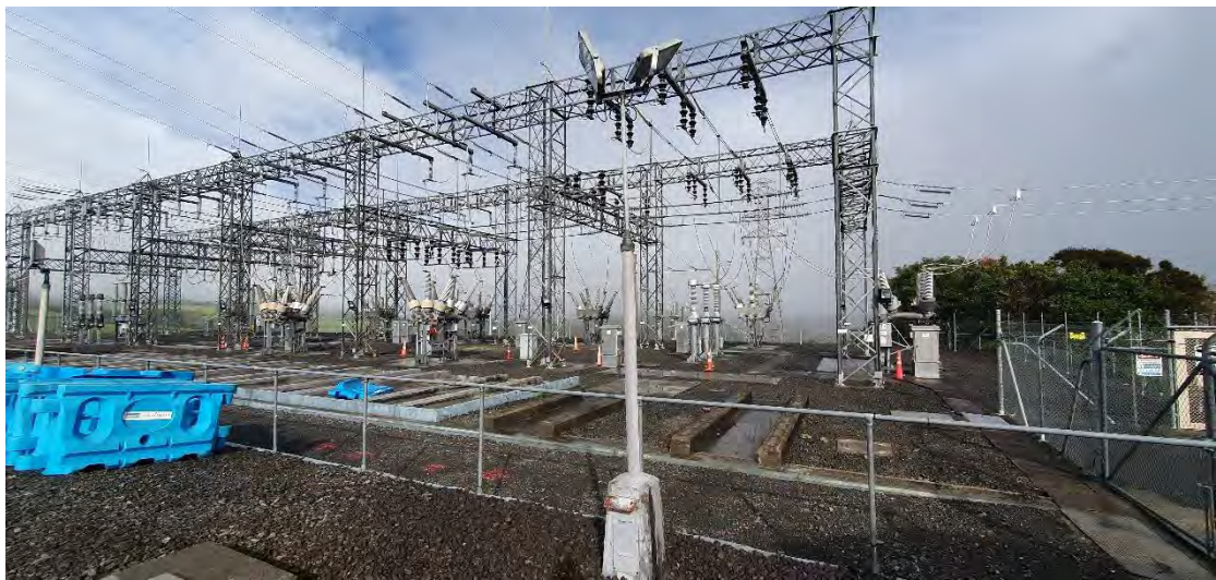
Figure 4: Existing Bombay Substation.
