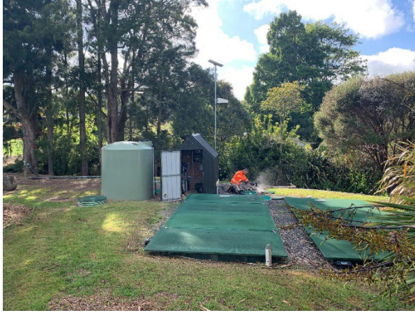
Figure 2-7: Flow balancing tanks, recirculation tank and treated effluent storage tank located on No.3 Denehurst Drive (Source: Aurecon)
