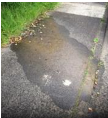
Groundwater on berm and footpath.
