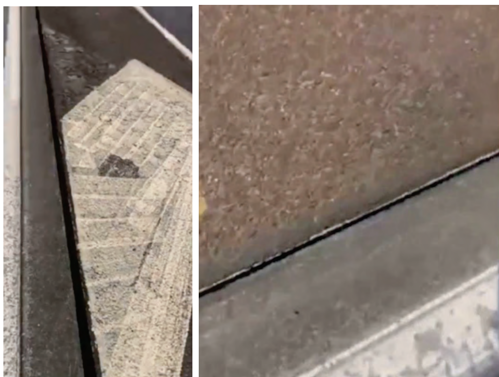
Figure 12 a \pm 50\text{mm} gap opening (left) and closing (right) on longitudinal joint between clip-on and main span. OIA 12397
