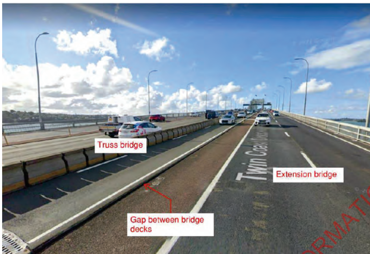
Figure 11 OIA 12397 Attachment 5 - location of joint observed to move under pedestrian loading
