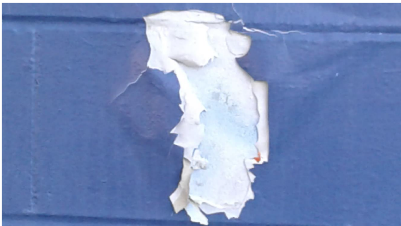
Paintwork flaking and peeling away due to water underneath
