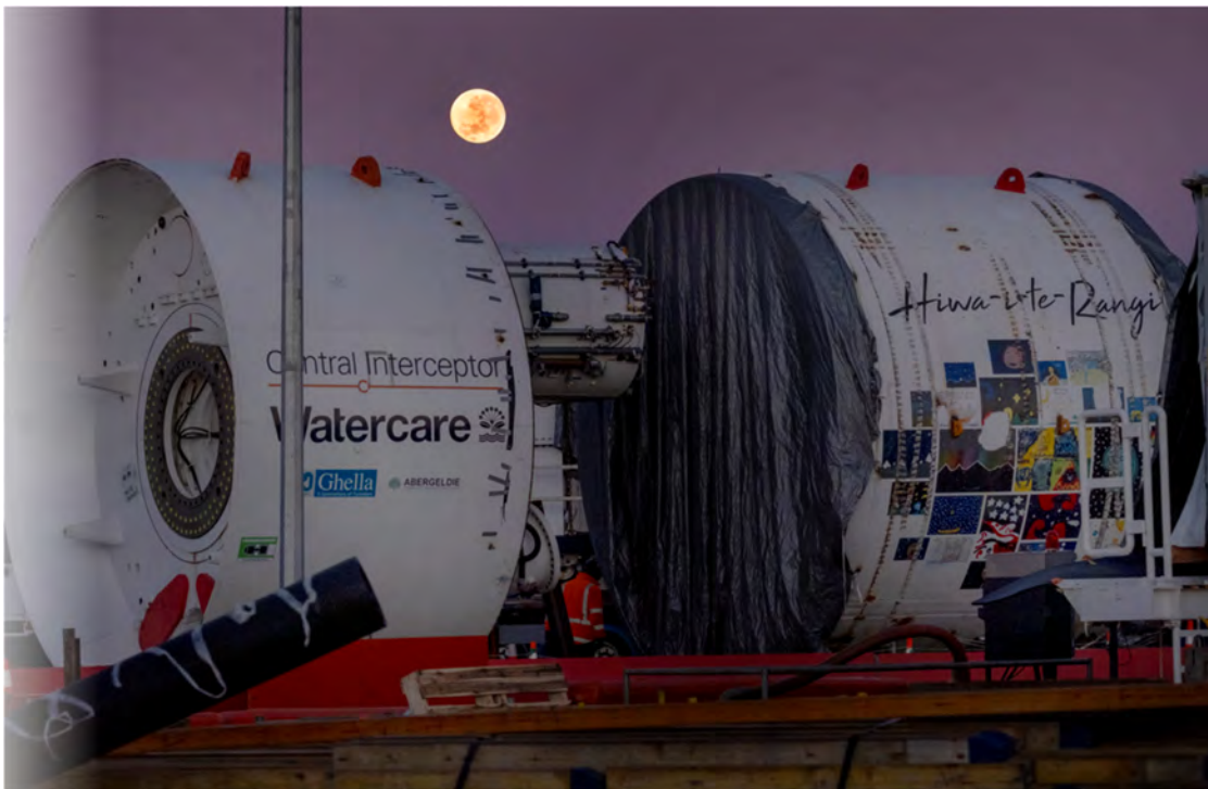
The moon over Watercare’s Central Interceptor Tunnel Boring Machine, named Hiwa-i-te-rangi. The TBM was named after one of the Matariki stars to which Māori would send their dreams or aspirations for the new year.
