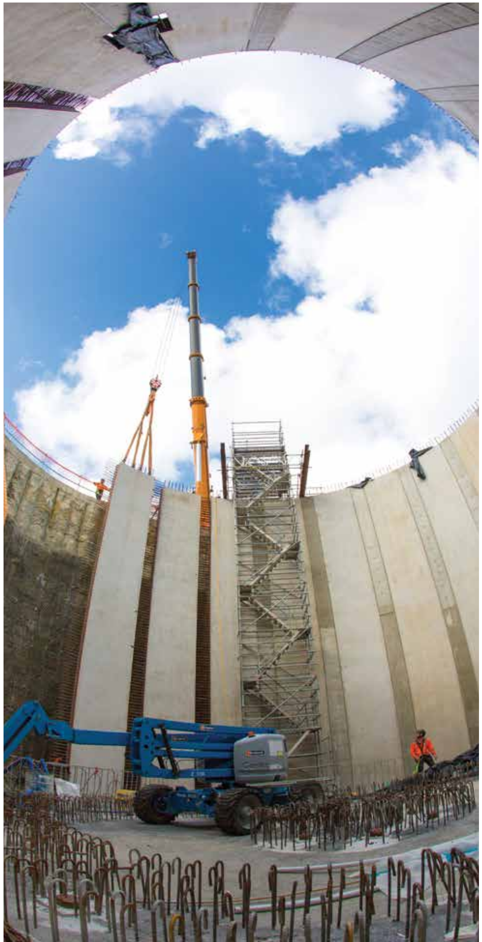
Watercare is constructing an underground storage tank in Madills Farm Reserve as part of a wider project to upgrade the wastewater network that services the east Auckland suburb of Kohimarama. The tank will improve beach water quality by reducing the frequency of wet weather overflows into the creek at Madills Farm Reserve.
