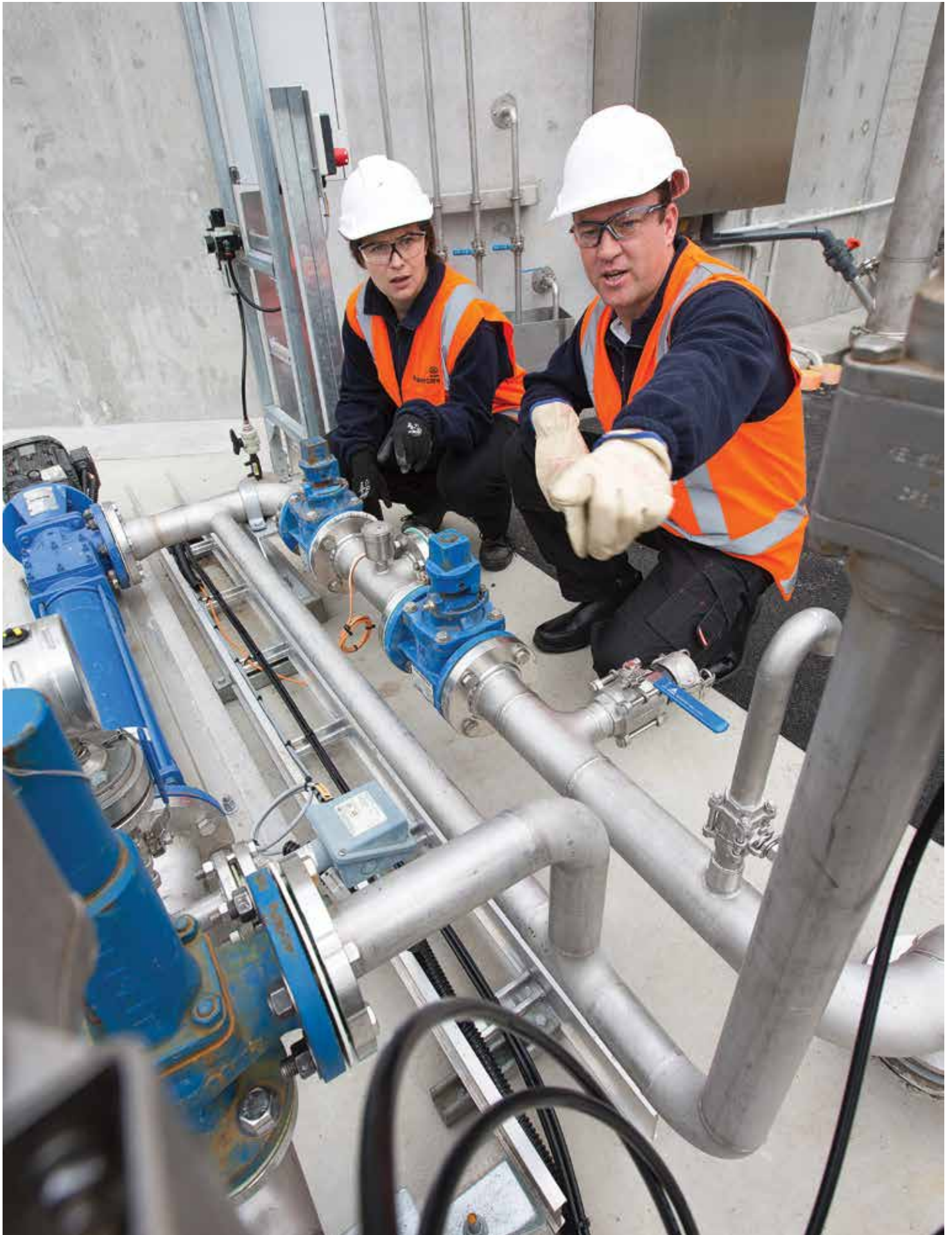
Water Supply Manager Nolwenn Lagadec discusses the new thickened sludge pump arrangement at Waikato Water Treatment Plant with Operations Controller Stuart Urquhart.
