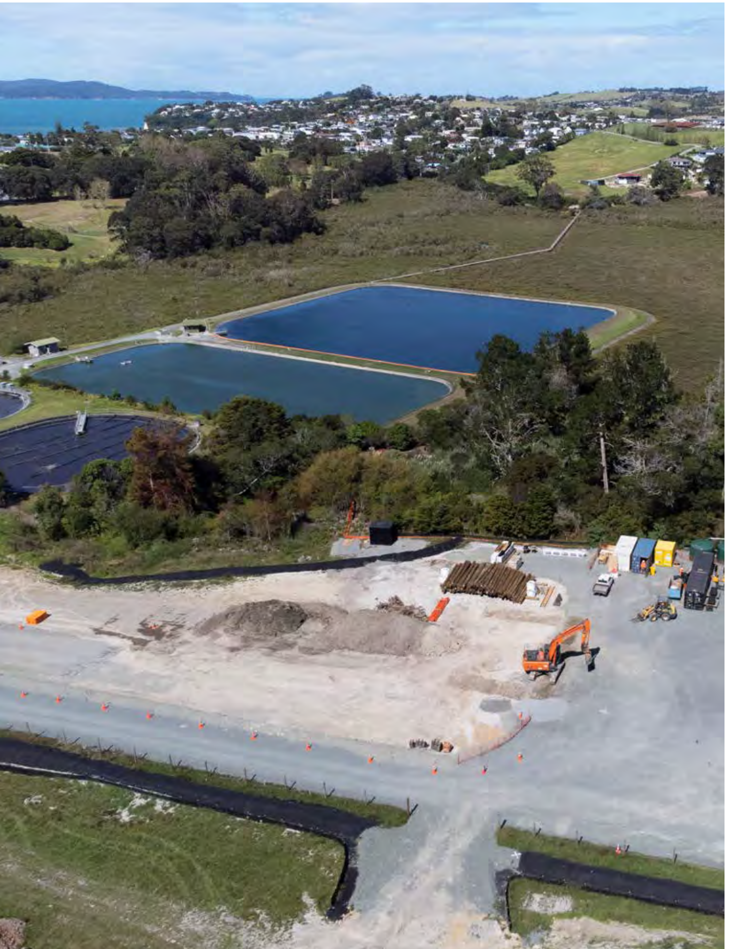
New wastewater plant at Snells Beach
