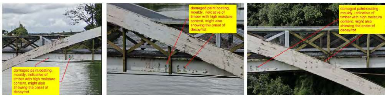
Figure 4: Conditions of the laminated timber main beams
