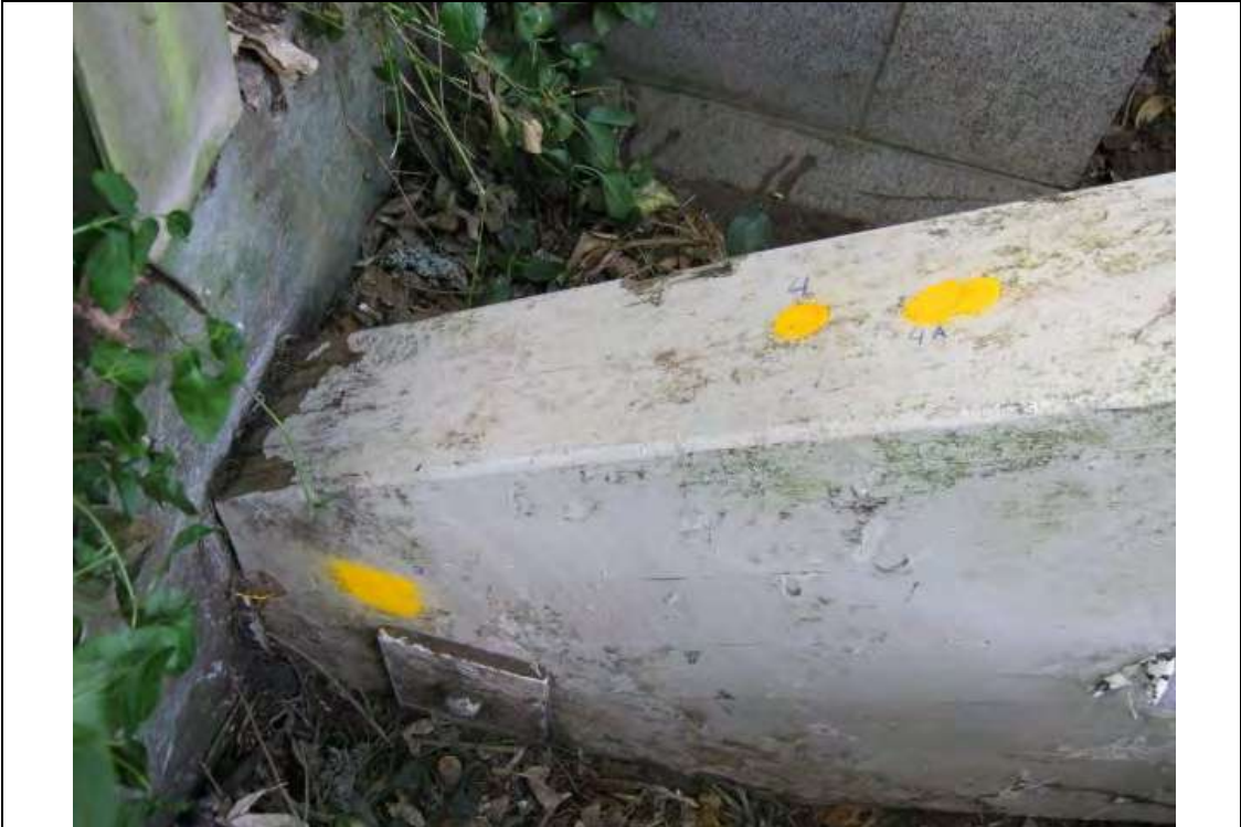
Probe #3 & #4 (#4A is the location of the "failed" probe) (Beam "B")
