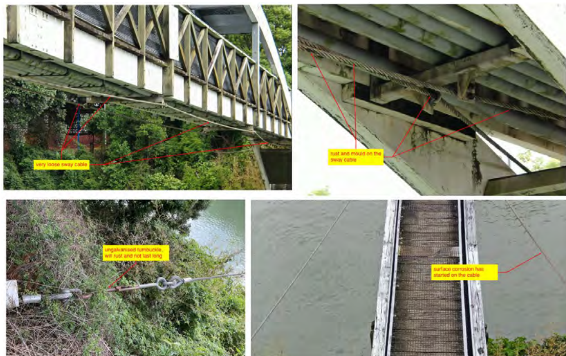
Figure 11: Conditions sway cables
