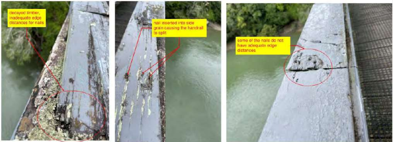
Figure 6: Conditions of the timber handrails and balustrades
