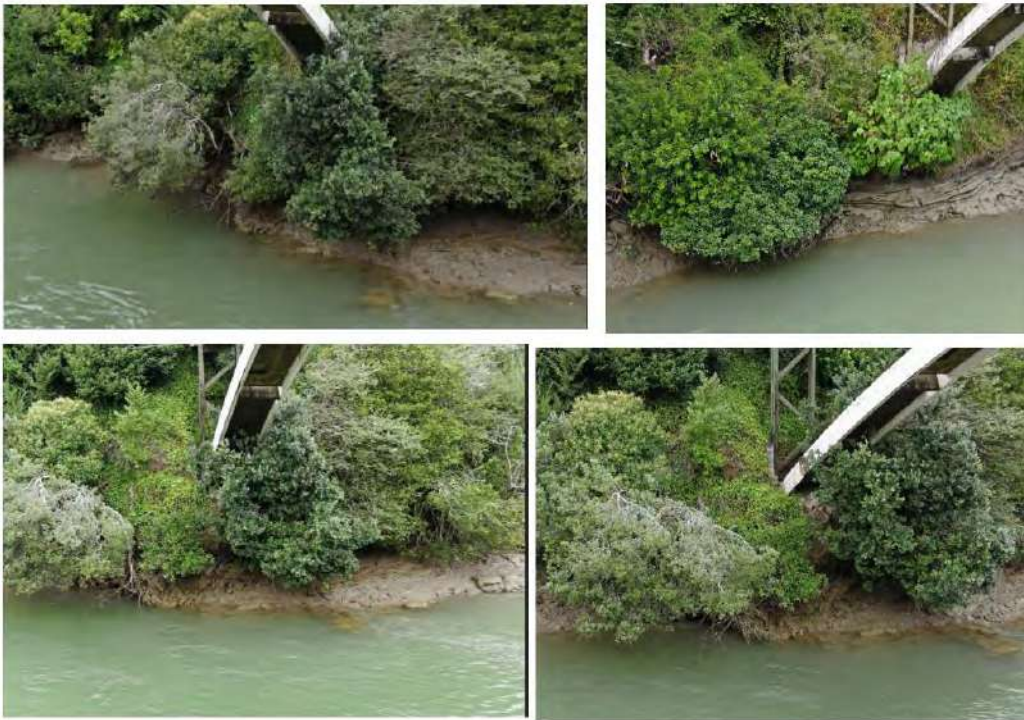
Figure 12: Conditions of the eastern bank of the bridge – Post Auckland flood event
