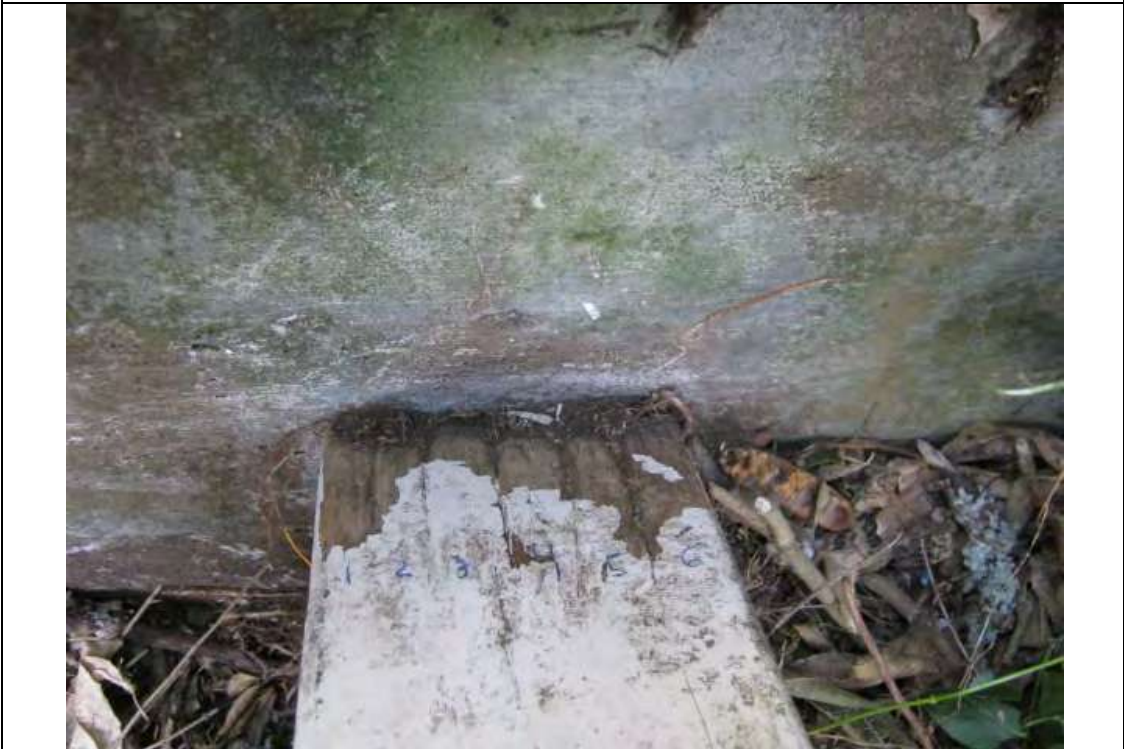
Photo showing the end of Beam "B" showing end decay and lateral de-lamination.
