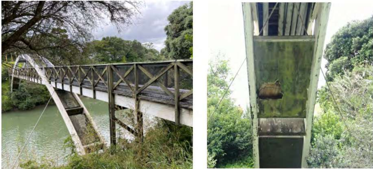
Figure 5: Conditions of the plywood diaphragms and box beams
