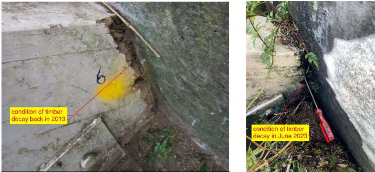
Figure 14: Side-by-side comparison of the base of the main timber arches on the Watene Rd side – Southern arches.
