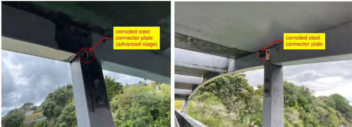
Figure 2a: Timber splits and corrosions at the hangers
