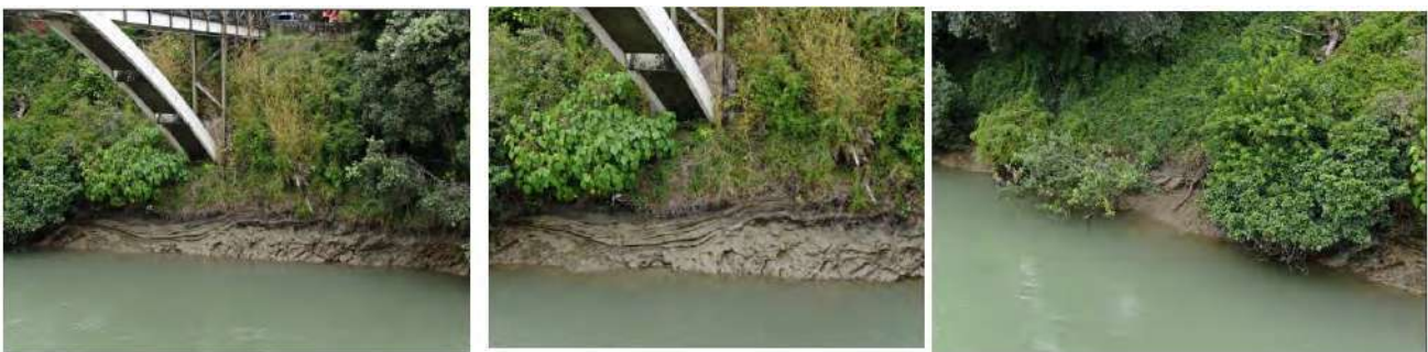
Figure 13: Conditions of the western bank of the bridge – Post Auckland flood event
