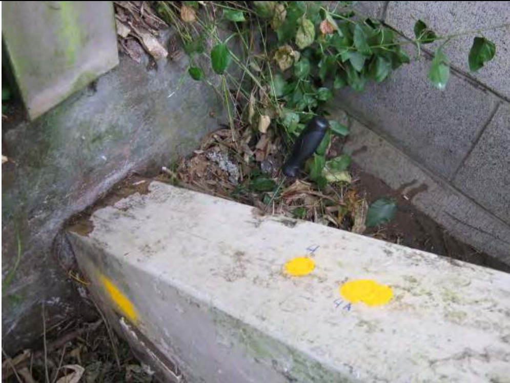
Photo showing Beam "B" with manual probe pushed into decayed wood.
