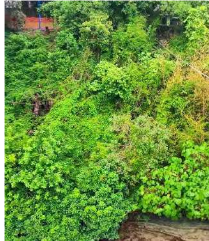
2. Steel cable obstructed by vegetation
