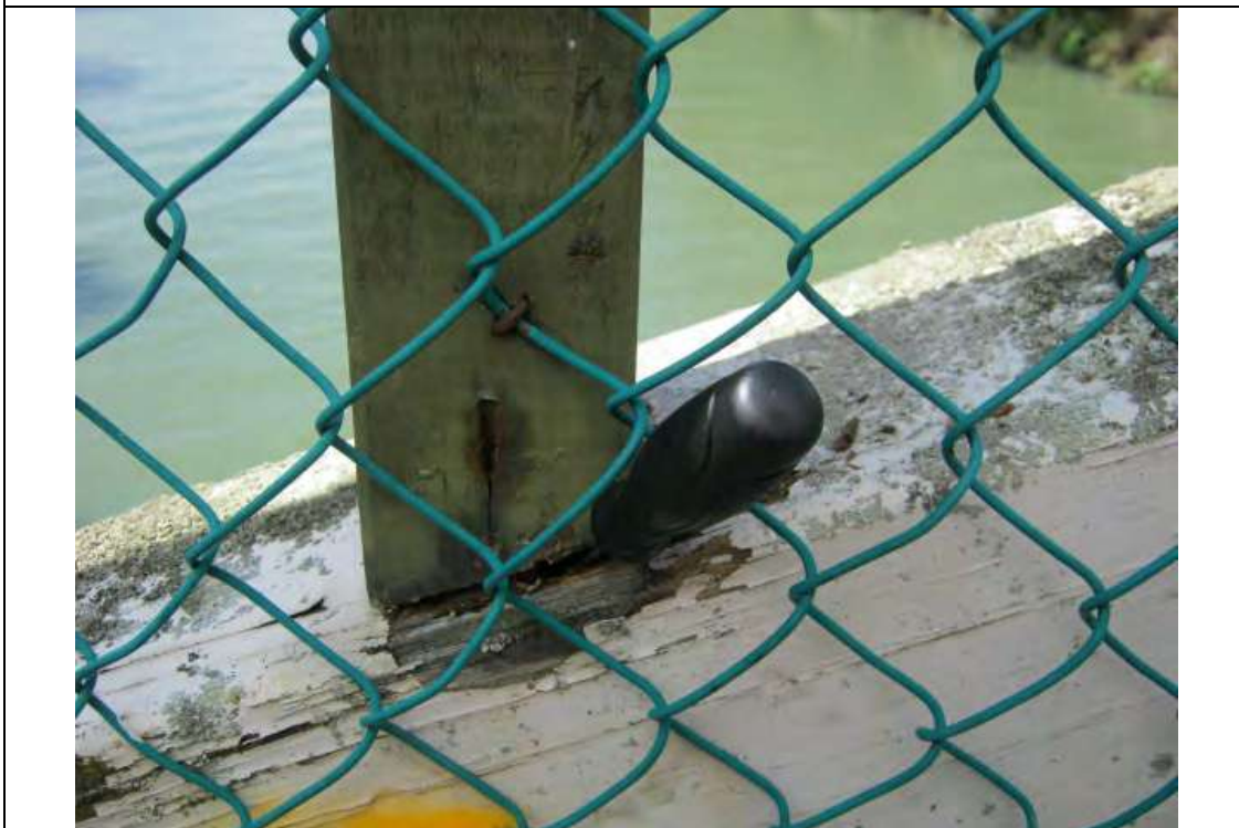
Severely decayed wood below handrail support (Beam "B"). 150mm manual probe completely inserted
