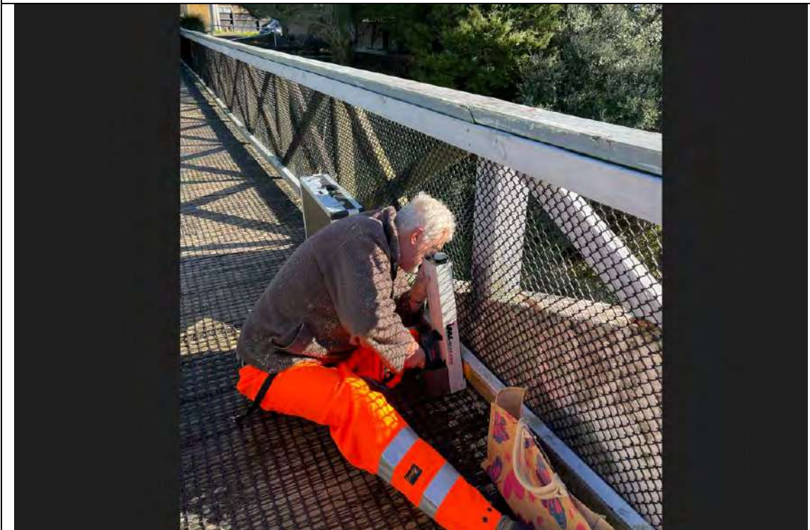
Photo showing the location of test drilling #3 The red arrow(s) depict the approximate drilling angle(s) Drilling was undertaken near vertical through the deck into horizontal beam
