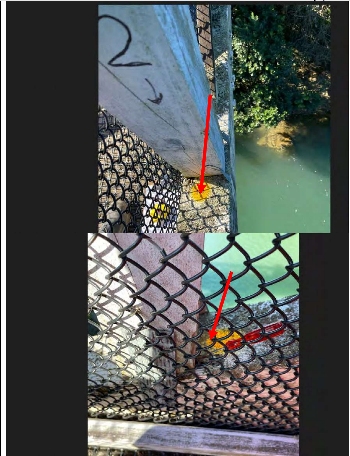
Photo showing the location of test drilling #2. The red arrow(s) depict the approximate drilling angle(s)
