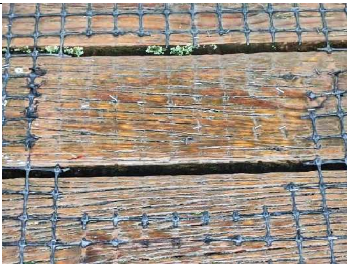
3. Typical: Damage to non-slip mesh
