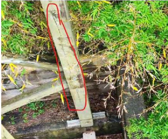
1. Timber piles show splitting
