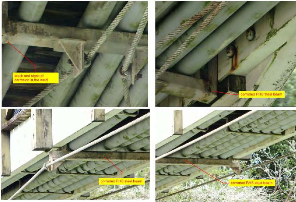
Figure 9: Conditions of RHS steel beams under the bridge
