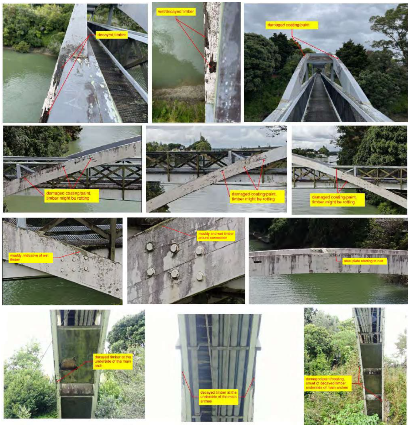
Figure 3a: Conditions of the laminated timber arches
