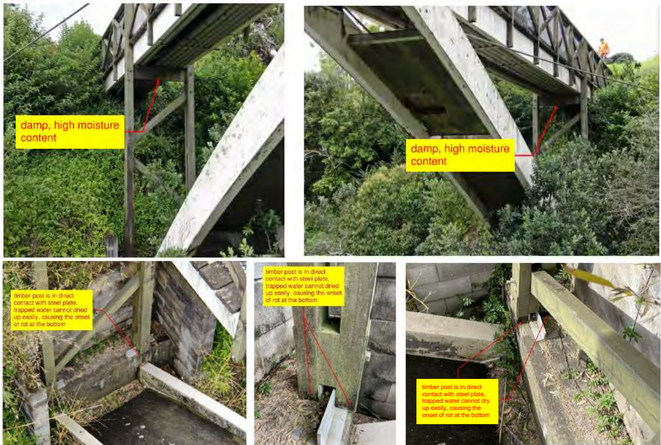
Figure 8: Conditions of the timber piers
