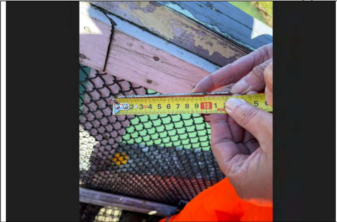
#2 severe decay detected under handrail post
