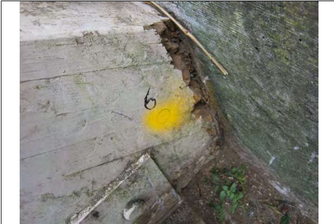
Photo showing beam "C", probe #6 and decay at beam end.
