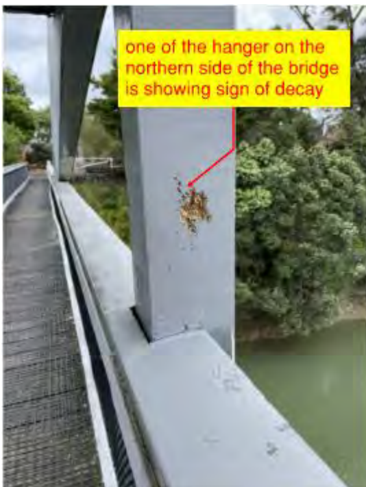
Figure 2b: Condition of one of the hangers on the Northern side.
