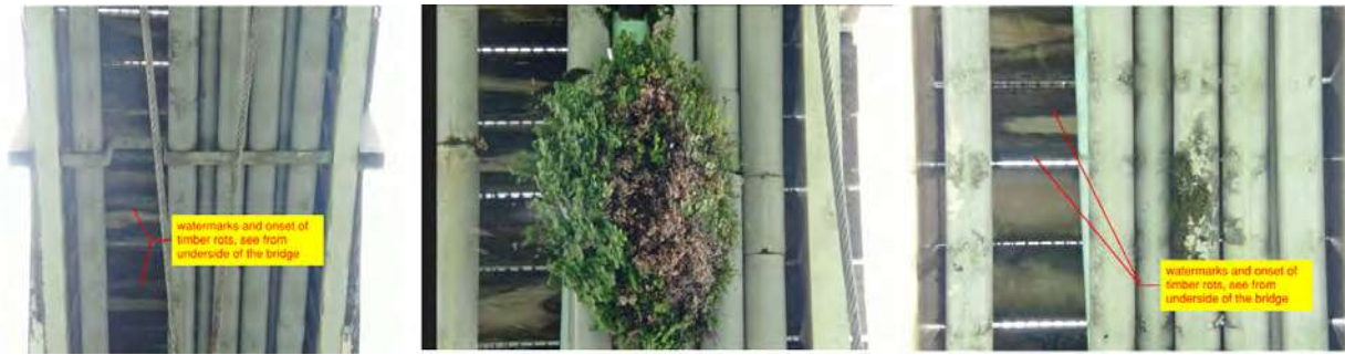
Figure 7: Conditions of the timber deck boards
