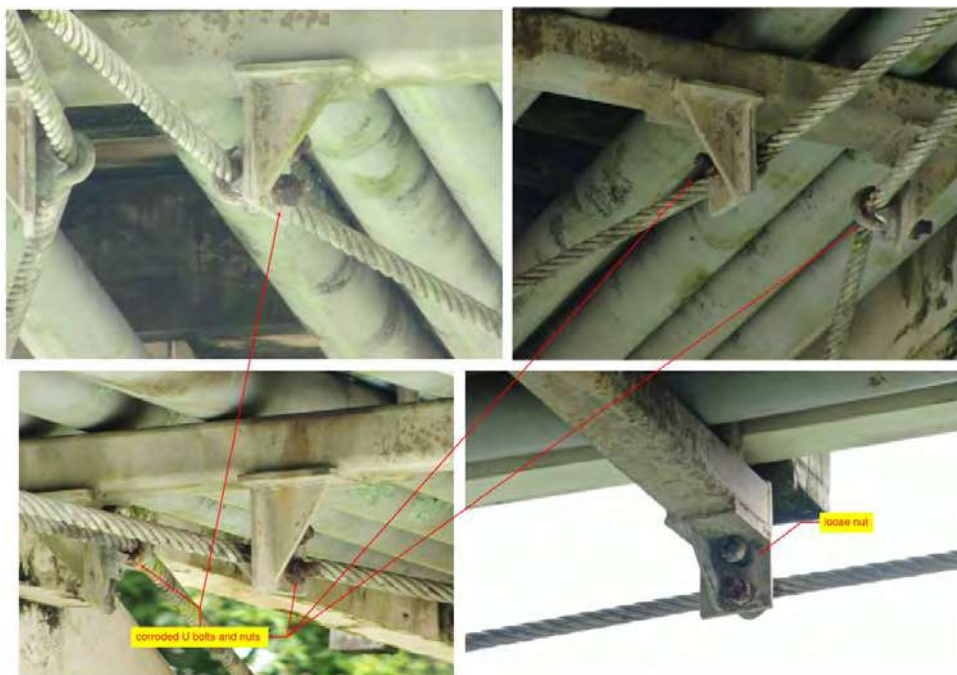
Figure 10: Conditions U bolts and nuts
