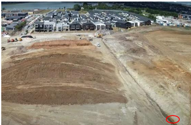
Unearthed groundwater found in the location shown.
