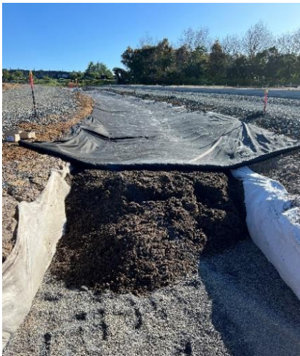
Rain garden in the centre of Joshua Carder Drive showing the gravel and soil mix layers, September 2022.
