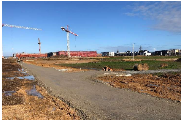
Recycled concrete used as sub-base under the shared path connection to Squadron Drive, June 2022.
