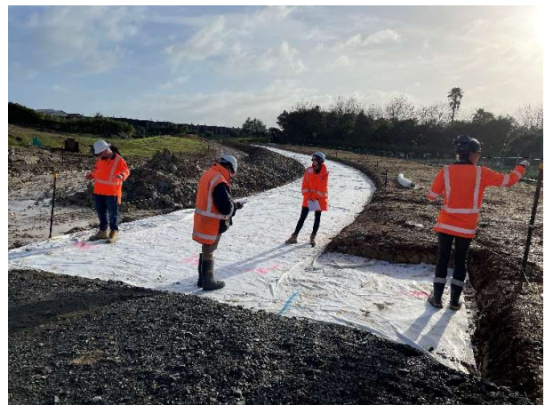
Filter cloth on Joshua Carder Drive under inspection before adding the sub-base, May 2022.
