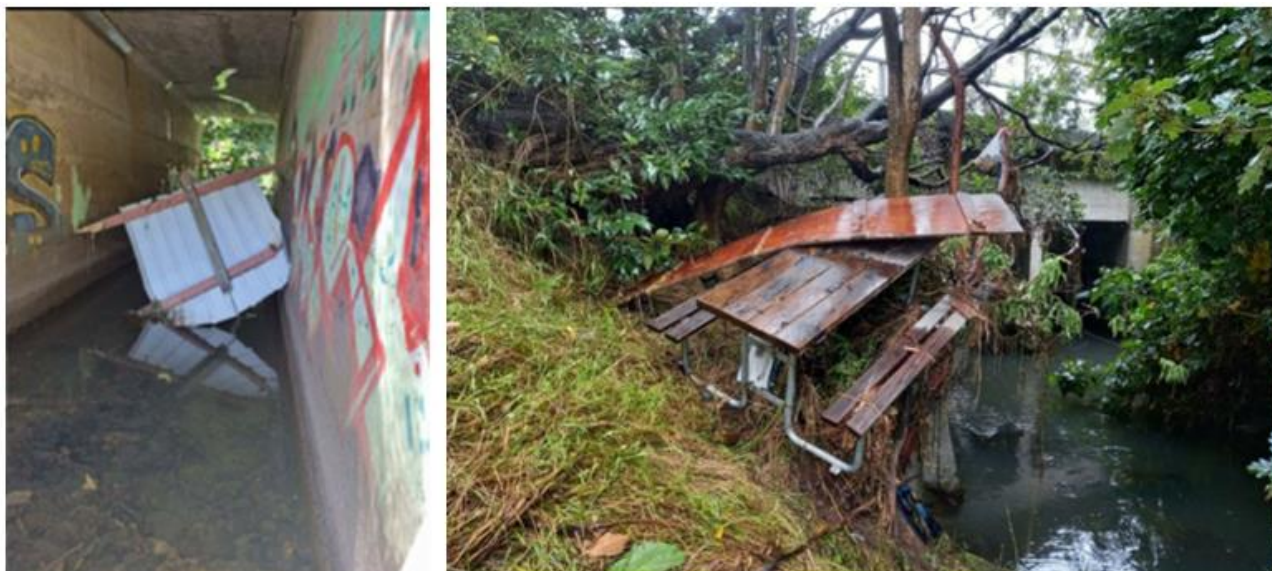
Figure 1-1: Debris caught in and around the existing Walmsley Road bridge culverts during the 2023 flood events - left-hand image shows a piece of fencing in within the culvert. Right hand image shows outdoor furniture in front of the culvert (source: Auckland Council Healthy Waters)
