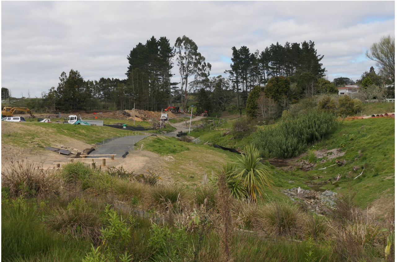
84 Hobsonville Road, Hobsonville (looking south towards Hobsonville Road, taken 9 Sept 2020 at 11.15 am)
