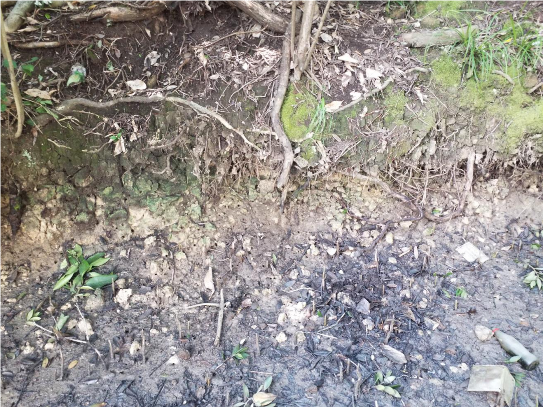
Figure 13: The typical toe of the slope observed onsite consisted of a vegetated bank composed of soft sediments with bioerosion evident.
