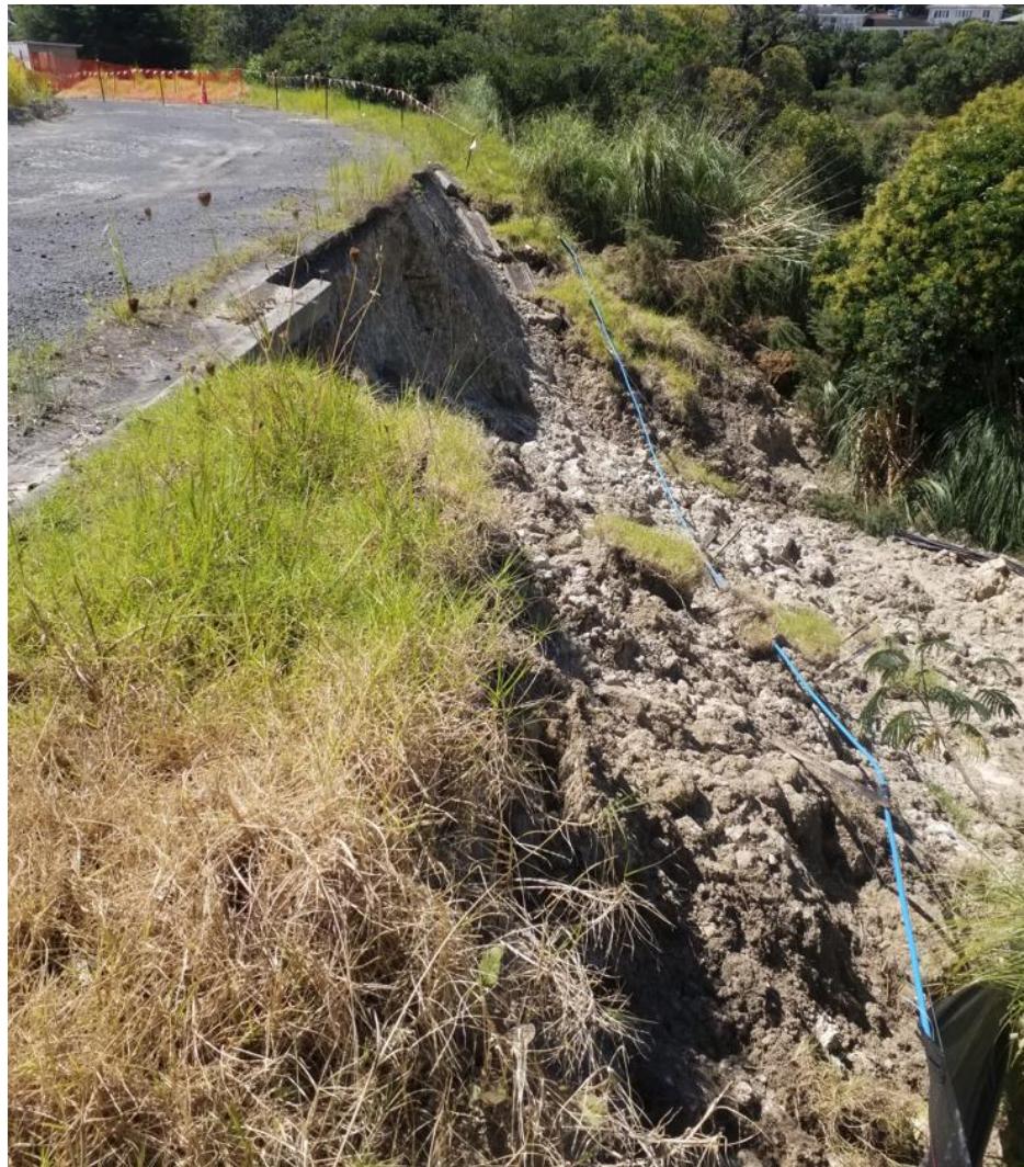
Figure 9: Slope instability visible during site visit
