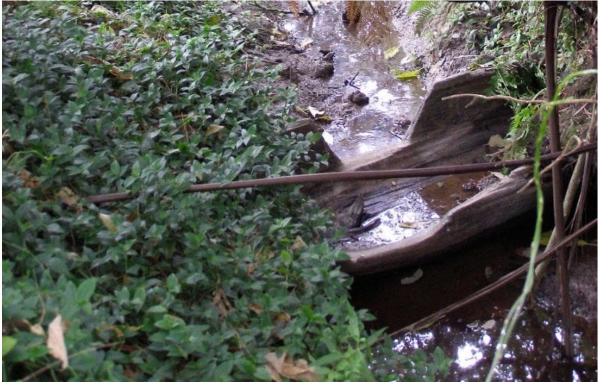
Figure 10: Photograph of the dam/sluice recorded at 60 Baker Lane (source: CHI no. 18372 site record)
