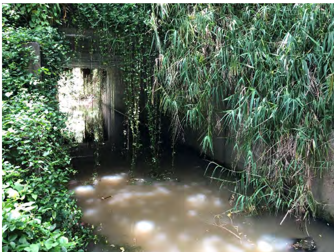
Figure 10-2 Under sized Waiarohia culvert
