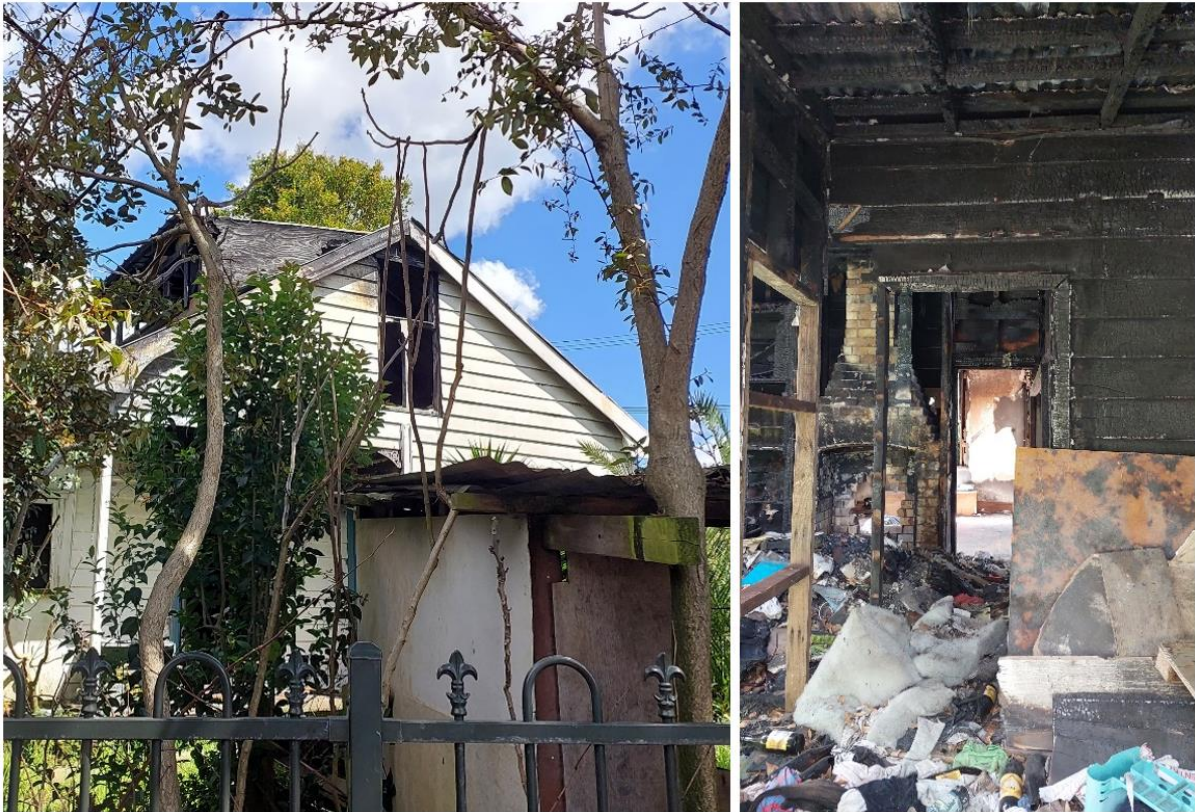
Figure 4 Unscheduled Recorded Built Heritage – Former Gardener's Cottage (CHI ref 2216) and landscaping to boundary
