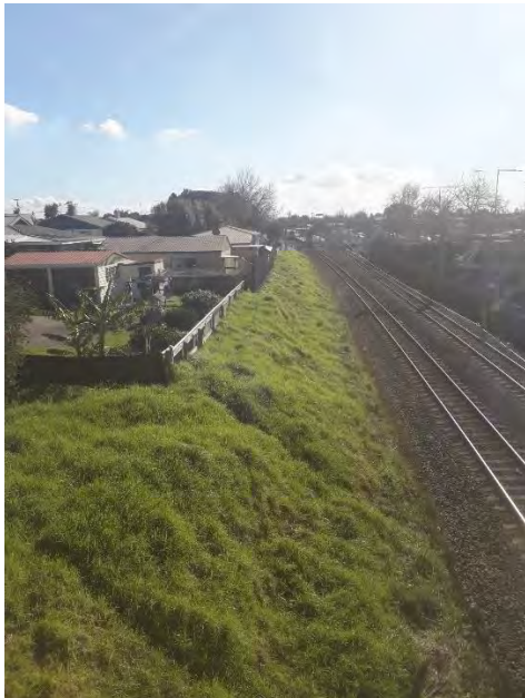
Photo 1 – Bridge Road Puhinui, looking north, site of Third Main and new retaining wall
