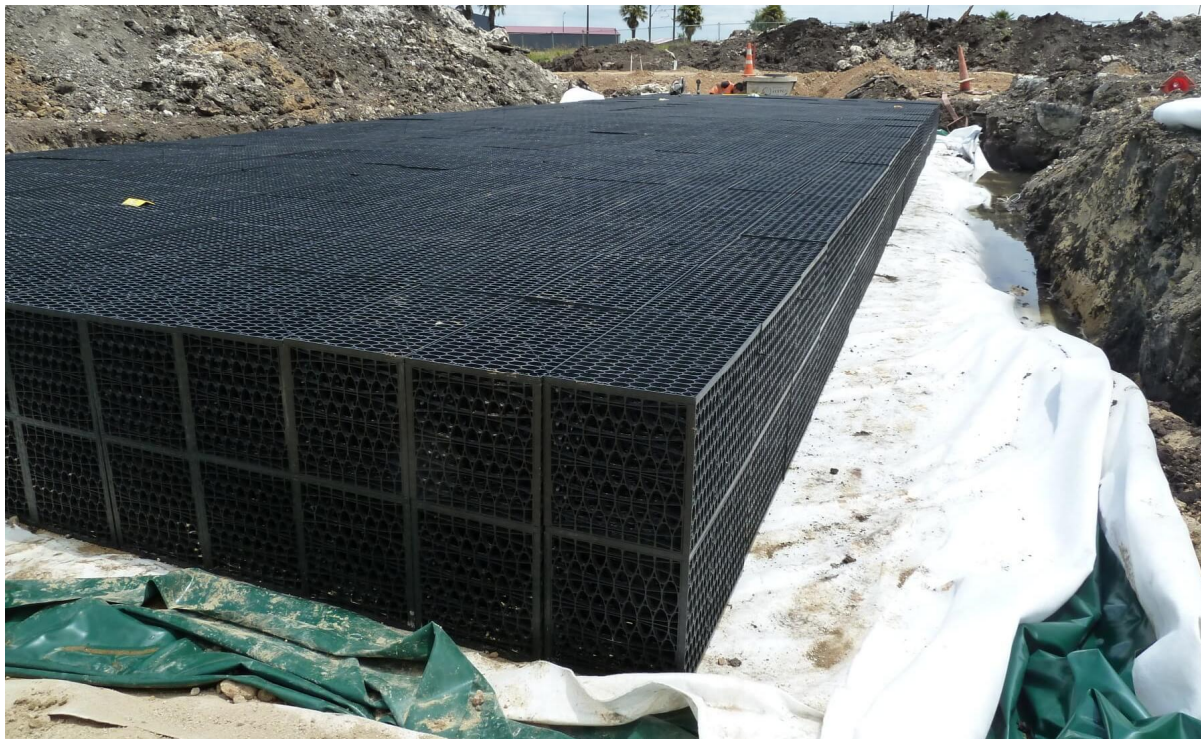
Figure 4: Installation of a large underground stormwater detention facility using a matrix of modular plastic cells that could be used on private lots
