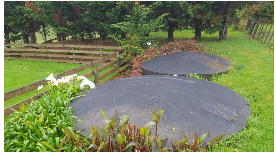
In-Situ Water Tanks
