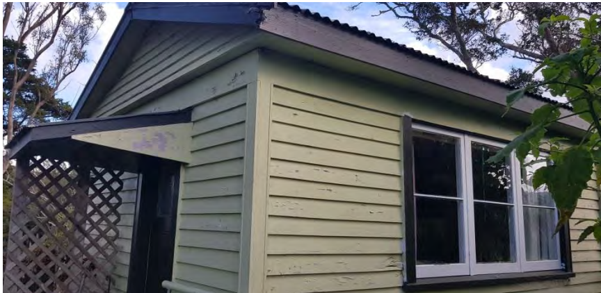
Minor Dwelling (PACM Soffits)
