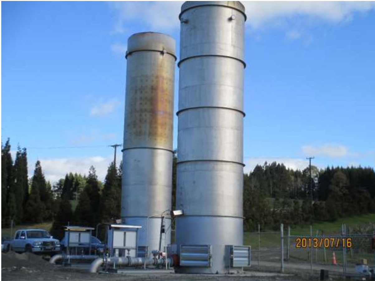
Figure 5.3: Flares at Redvale Landfill
