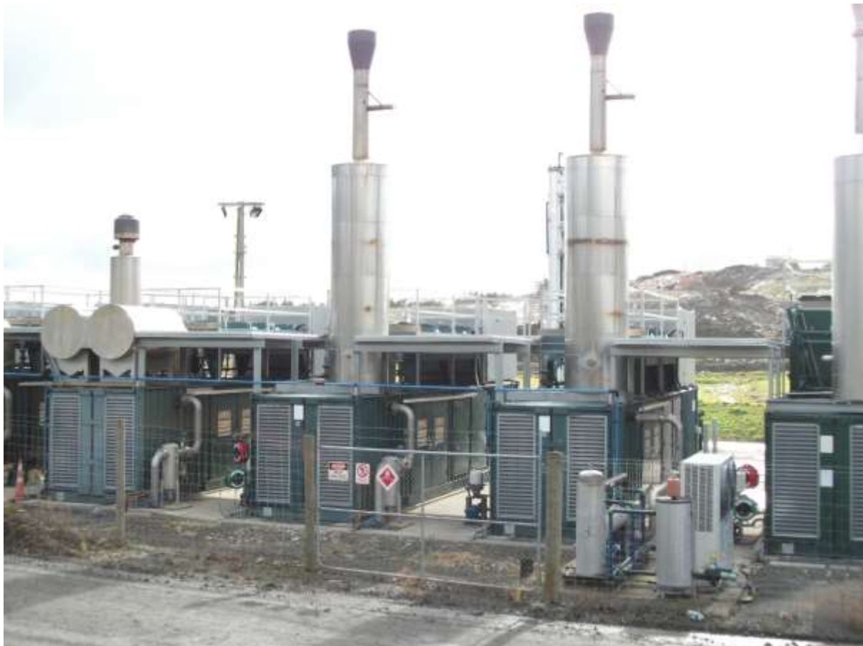
Figure 5.4: Photograph of generators at Redvale Landfill
