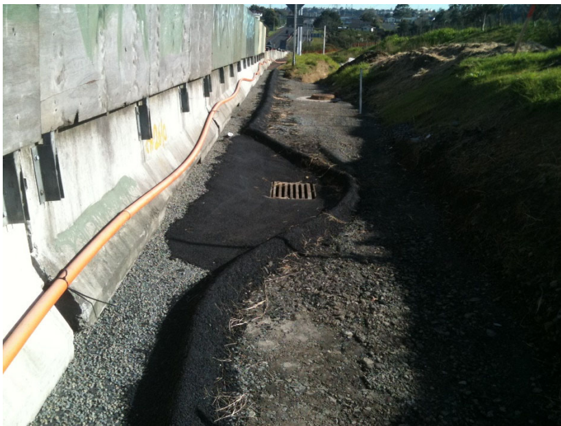
Photo 2: Hotmix Bund used to divert existing road runoff and separate works area, used on the North-Western Motorway.
