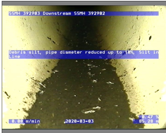
Photo: 1_11A 85.28m, Debris silt, pipe diameter reduced up to 10% / Silt in Line
