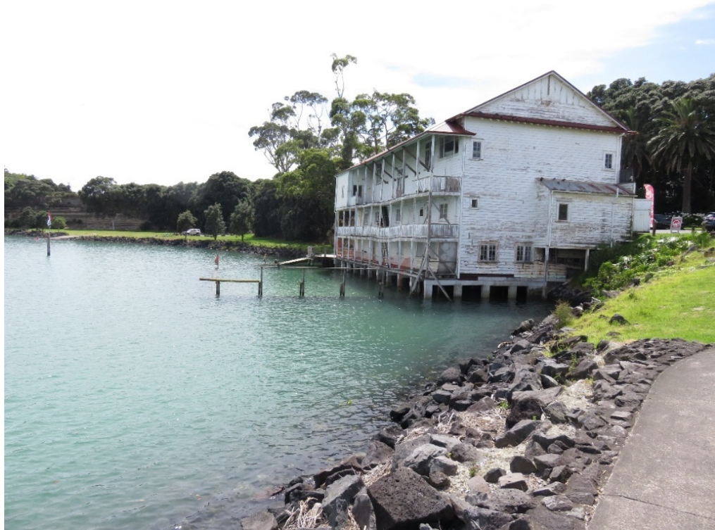
Figure 6: The three storey former Bayswater Yachting Club building on Sir Peter Blake Parade.
