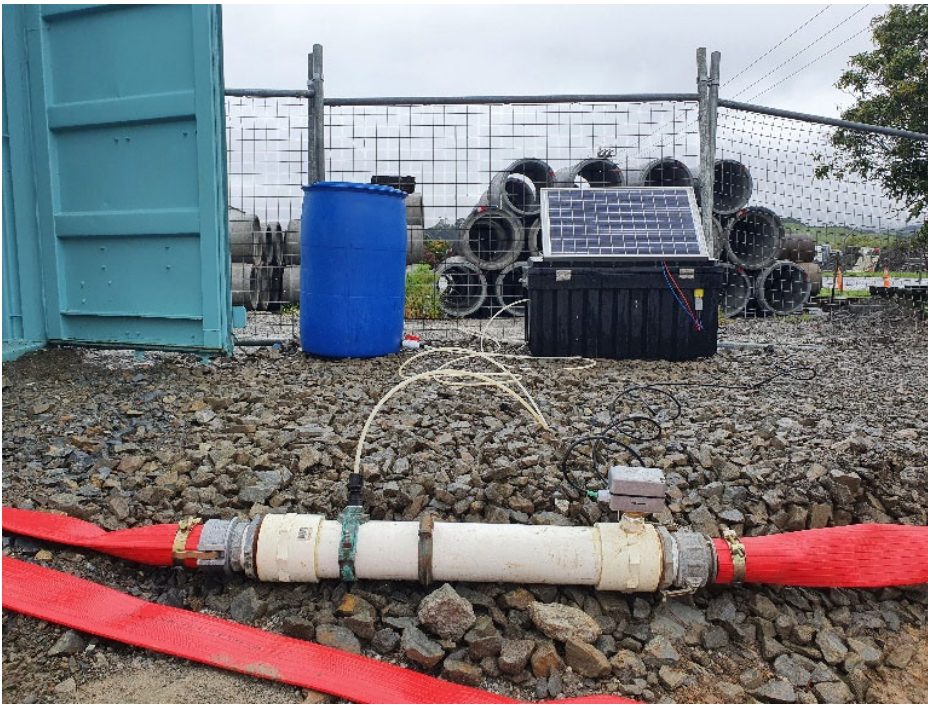
Figure 4: Example of an in-line electronic chemical dosing system (Source: Erosion Control).
