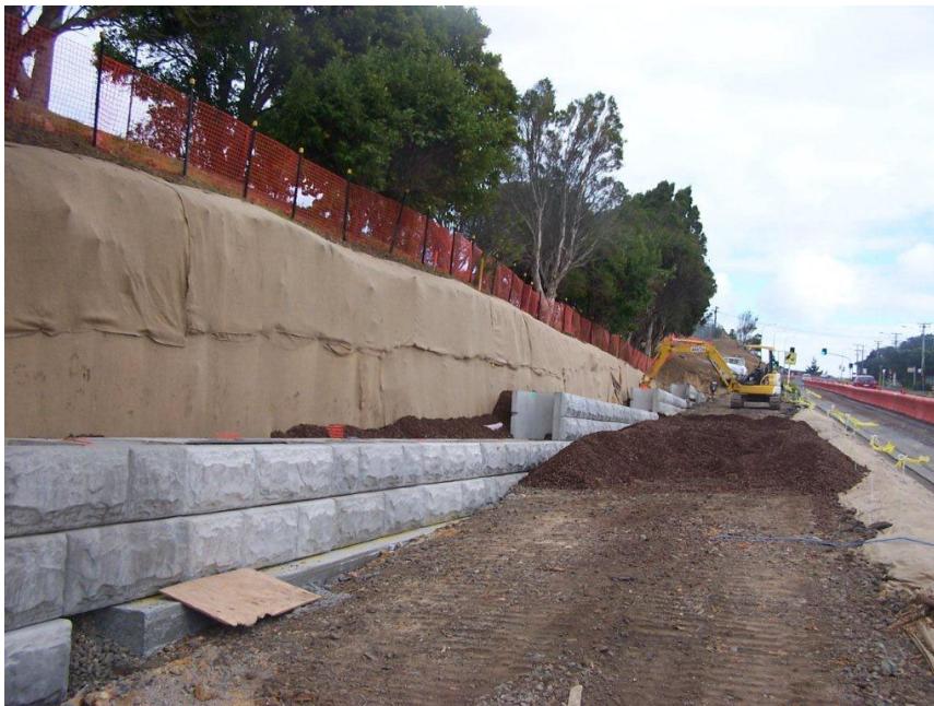
Figure 4 Rapid stabilisation, cut and cover (geotextiles and aggregate) used on the Albany Highway project
