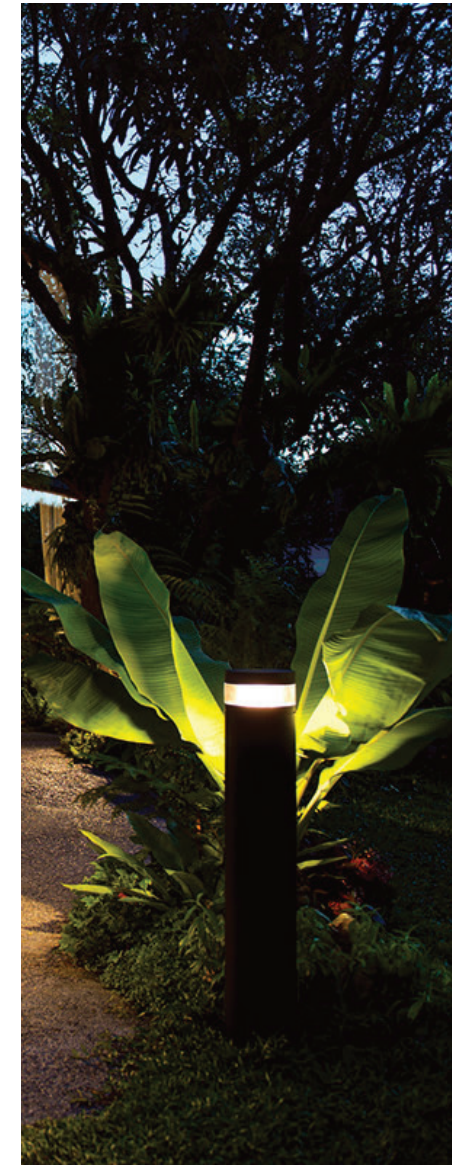
ACCESSWAY AND BOARDWALK EDGE LIGHTING
