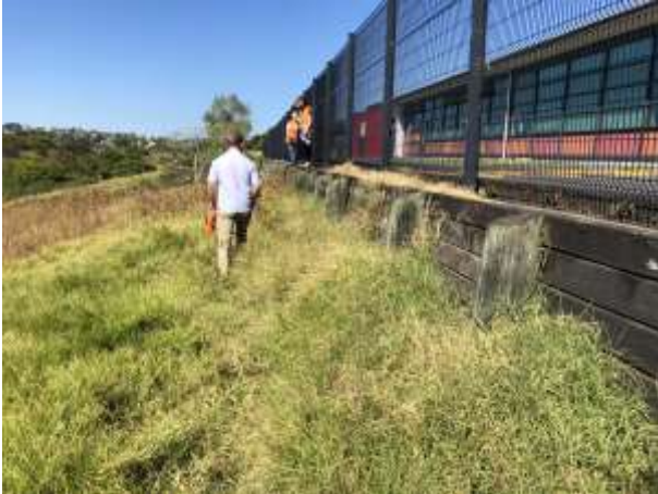
Evidence of existing retaining wall along northwest boundary in northern portion of the site supporting accessway. High permeability fences at boundary.
