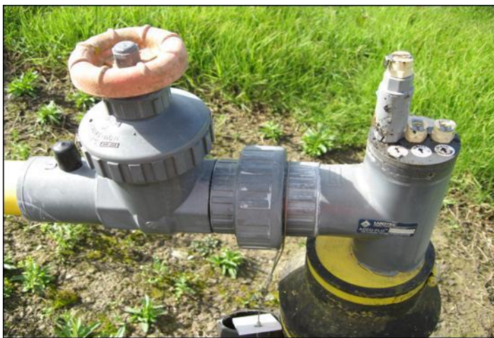
Figure: Landfill gas well head
