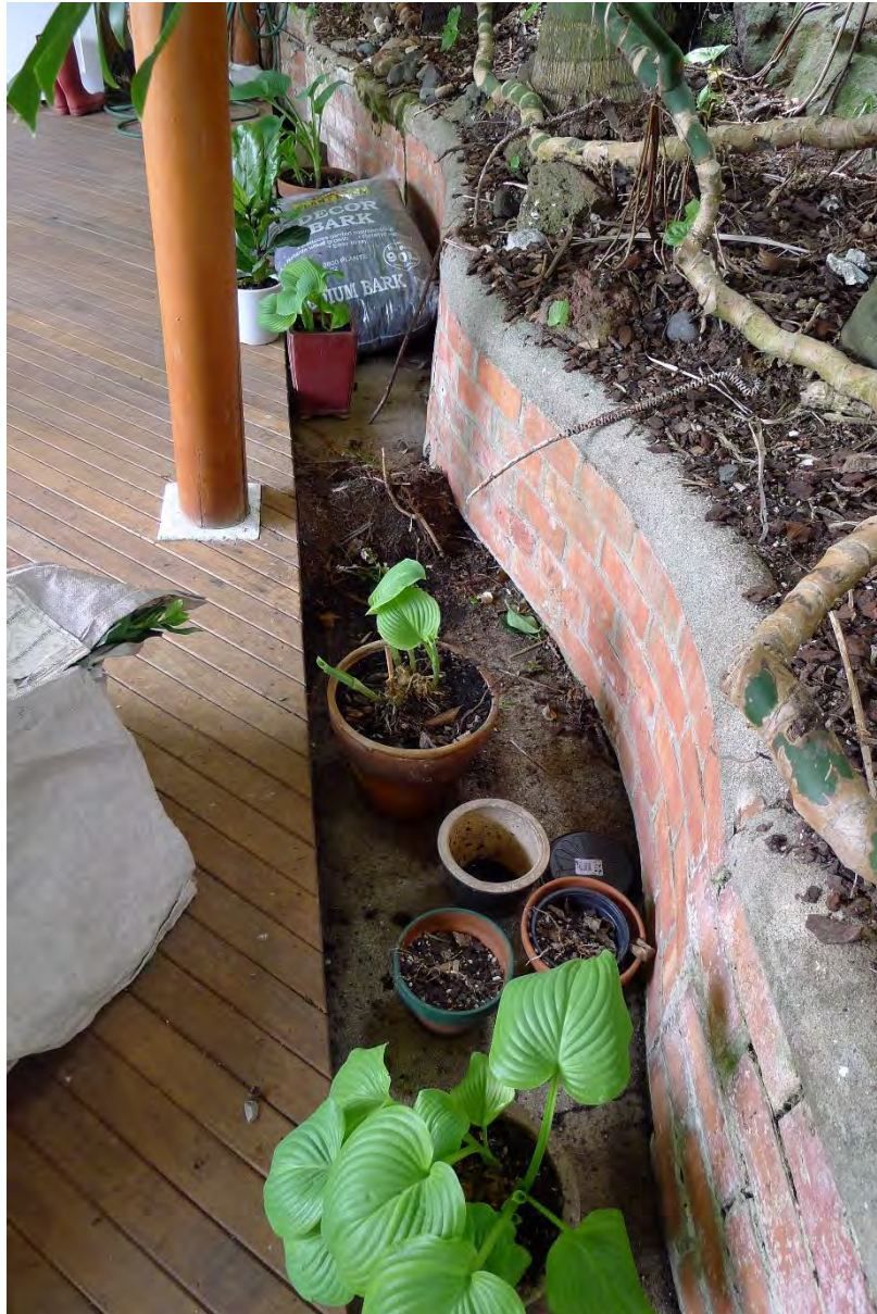
Figure 24. Brick retaining wall and concrete path (partially decked over) at the foot of the escarpment (visible top right). The spring cavity reportedly underlies these structures. Auckland Council photograph 21 October 2020.
