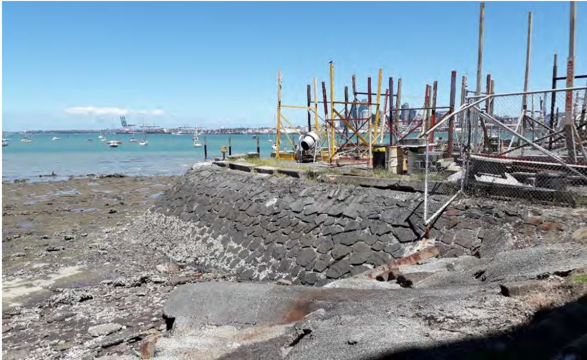
Figure 82: Northcote Point Sea Wall, including sea wall at "The Gold Hole" (David Bade, Auckland Council, 15 December 2020).
