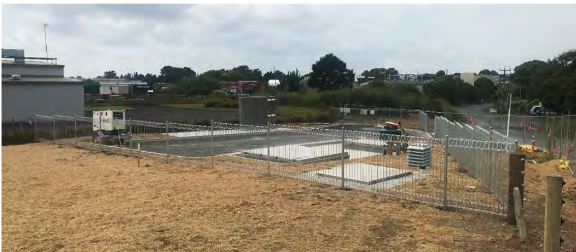
Plate 5. Example pump station, Flanagan Road Pump Station in Drury.
