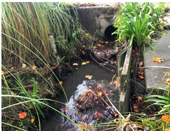
Photo 29. Watercourse 25 drained through a culvert with a vertical drop at the concrete apron.
