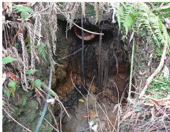
Photo 55. A tall drop was present within Watercourse 38 acting as a barrier to fish passage.
