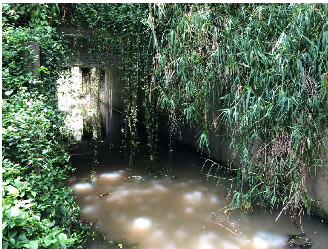
Figure 10-2 Under sized Waiarohia culvert
