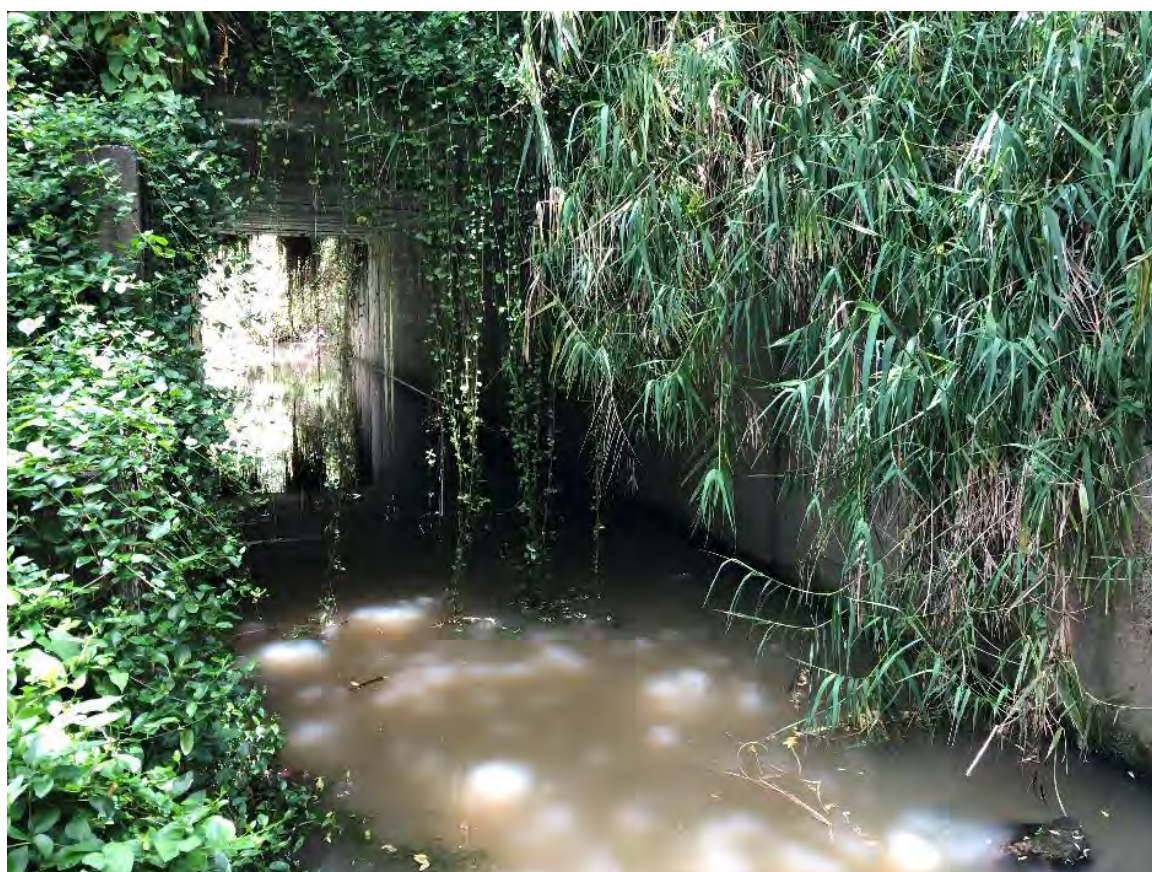
Figure 10-2 Under sized Waiarohia culvert
