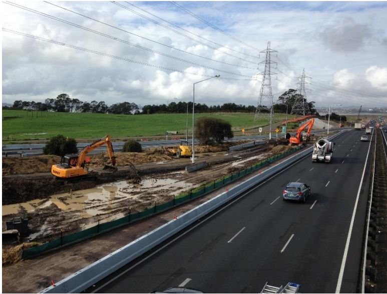
Photo 3: Silt Fences used to treat construction water, used on the North-Western Motorway.
