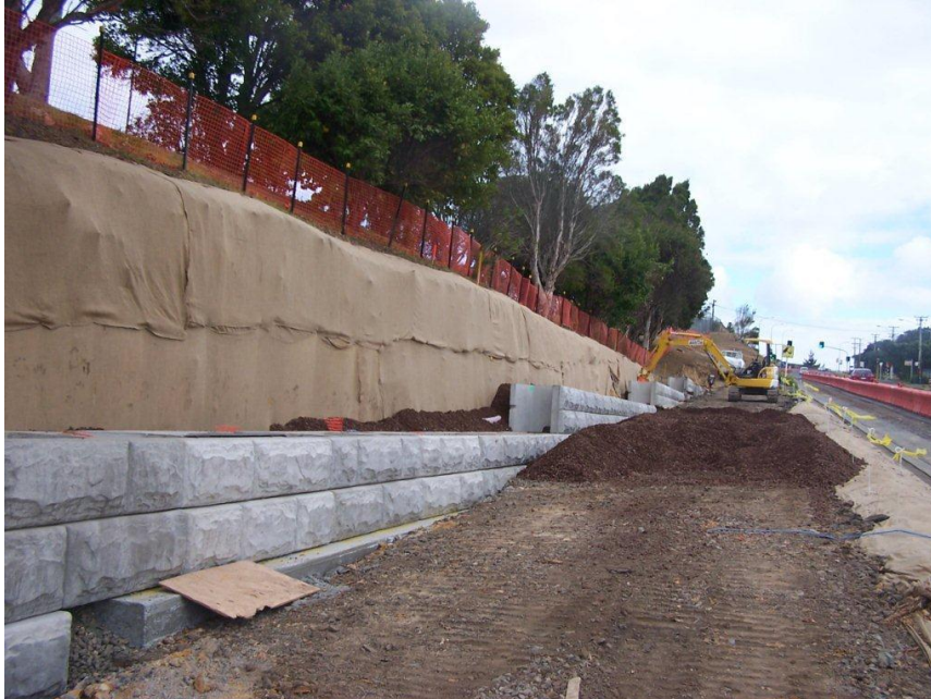
Photo 1: Rapid stabilisation, cut and cover (geotextiles and aggregate) used on the Albany Highway project
