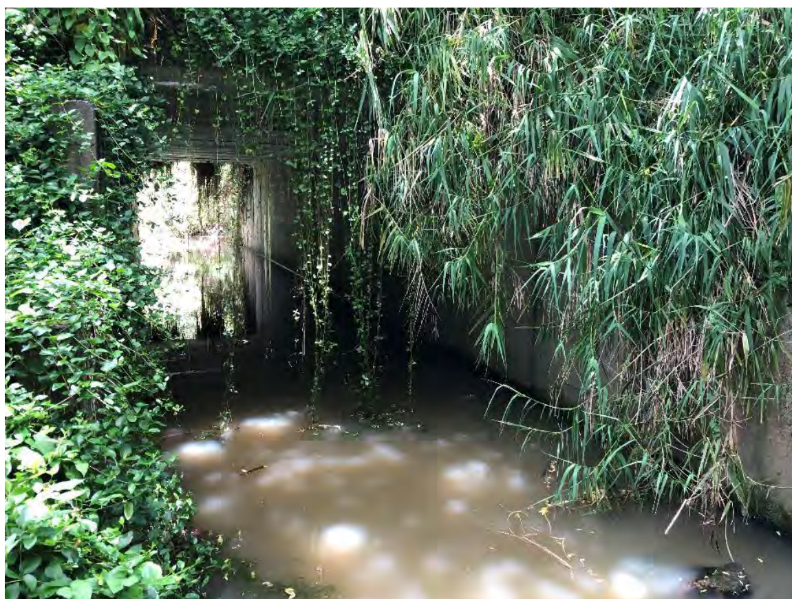
Figure 10-2 Under sized Waiarohia culvert
