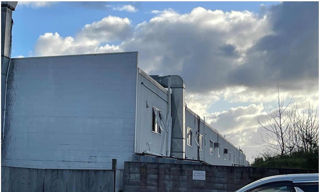
Figure 20. North-facing walls of commercial buildings at 2-202 Torrens Road (location C); photo taken from east end of buildings looking west, 16 May 2023.
