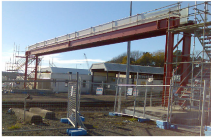
Temporary pedestrian overbridge – providing construction access across Ti Rakau Drive for the Reeves Road Flyover
