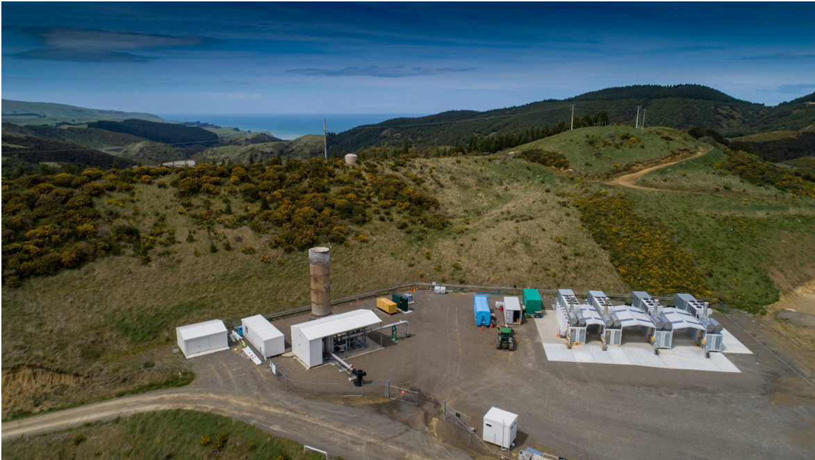
Above: Gas Plant
