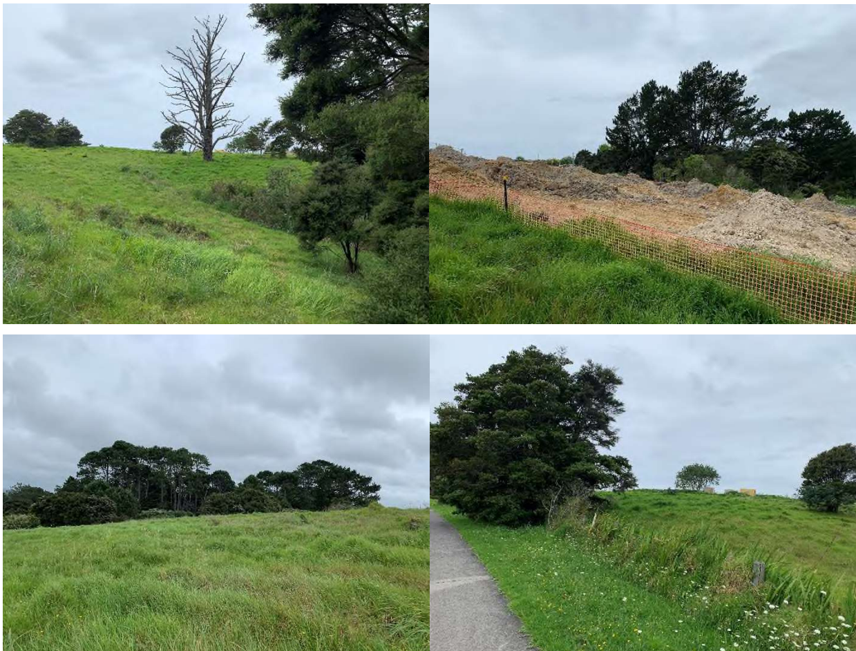
Image 1 (Top Left). Head of Western Gully looking North. Image 2 (Top Right) Vegetated Head Scarp along the eastern site boundary, with earthworks upslope looking Northeast. Images 3 and 4 (Bottom) Gently sloping ground within the central and northern portion of the site.
