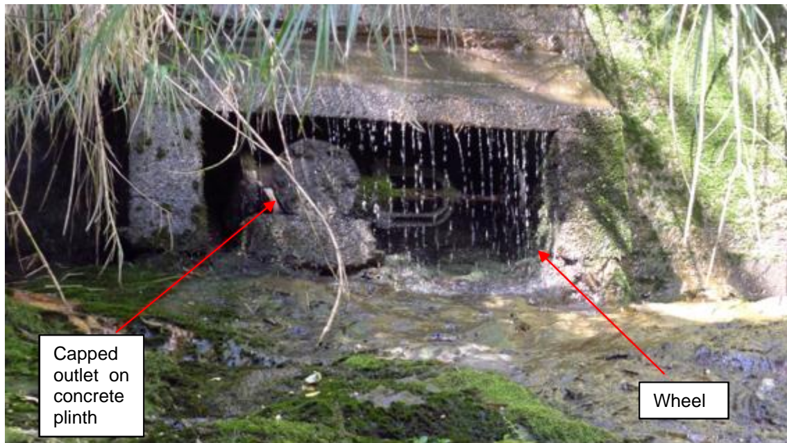
Figure 11. Outlet valve at base of dam. The pipe attachment flange has been capped with a metal plate, indicating that the pipeline was dismantled and removed upon decommissioning.
