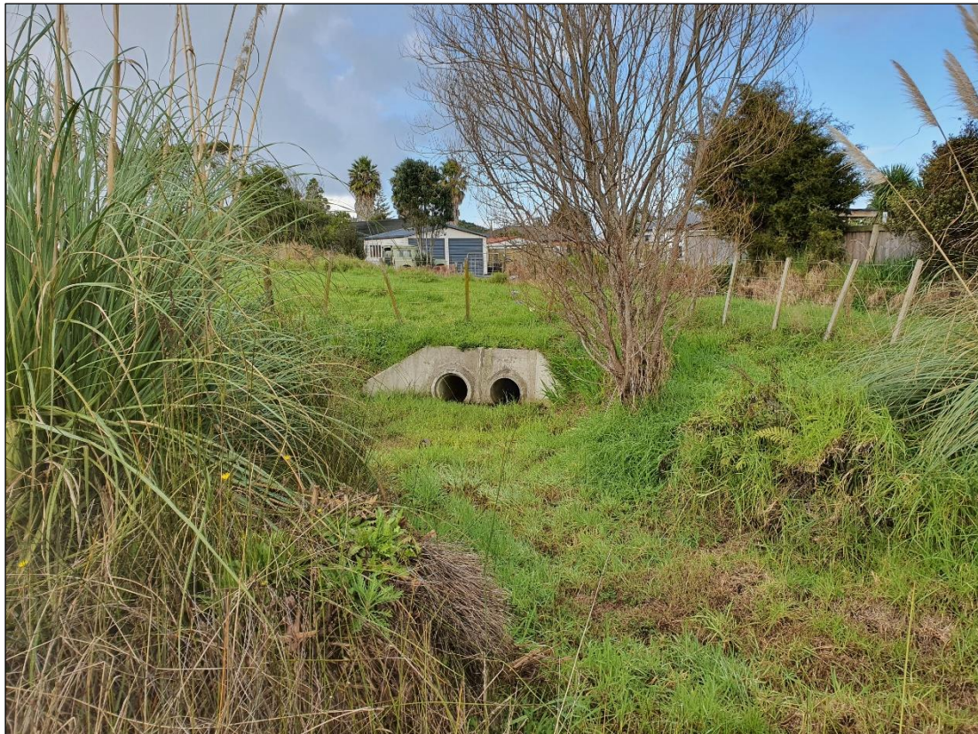
FIGURE 7: Dry detention pond outlet.
