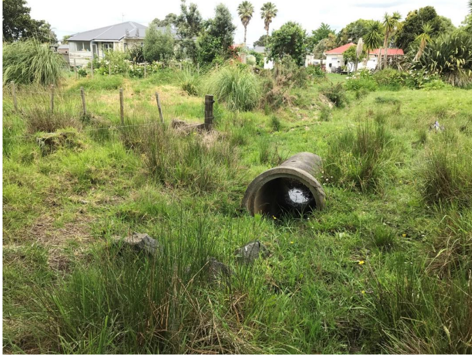
Photograph 3: Water pooled in culvert in southern corner of site.
