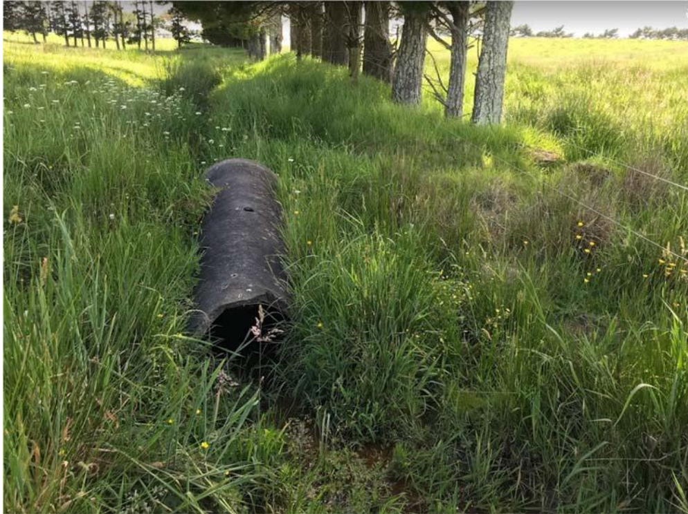
Photograph 7: Looking north at A3, with W3 on the right of the photo. The channel levels out, so high flows will overflow into W3.
