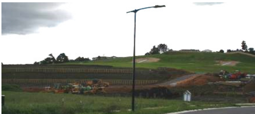
Photograph 5: New residential areas under development in the John Andrew Drive area. Note the need for extensive retaining in this moderately sloping topography.
