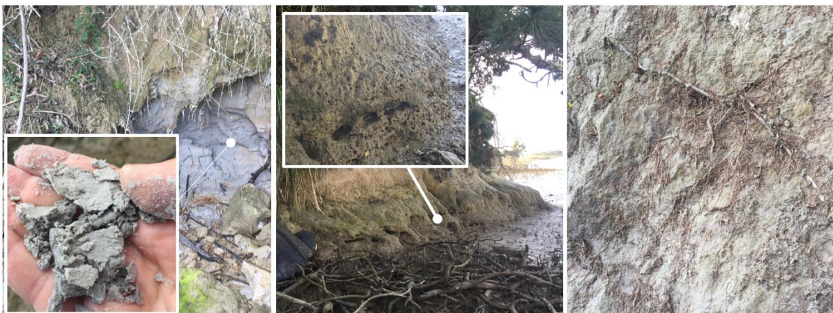
Figure 3-6 Surface weathering, bio-erosion and root pressure
