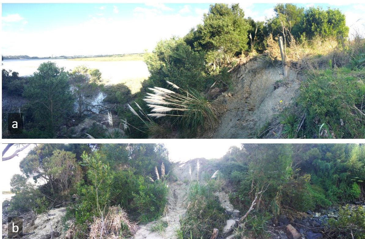
Figure 3-7 Instability within Cell A PF exposures (Photo top and bottom taken at the same location)
