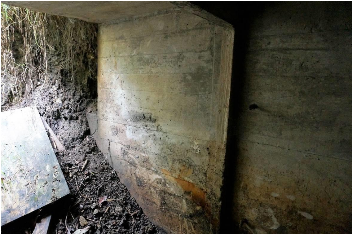
Figure 26. Looking out (NW) from within the ammunition recess in the central emplacement, showing side wall inside and outside the recess
