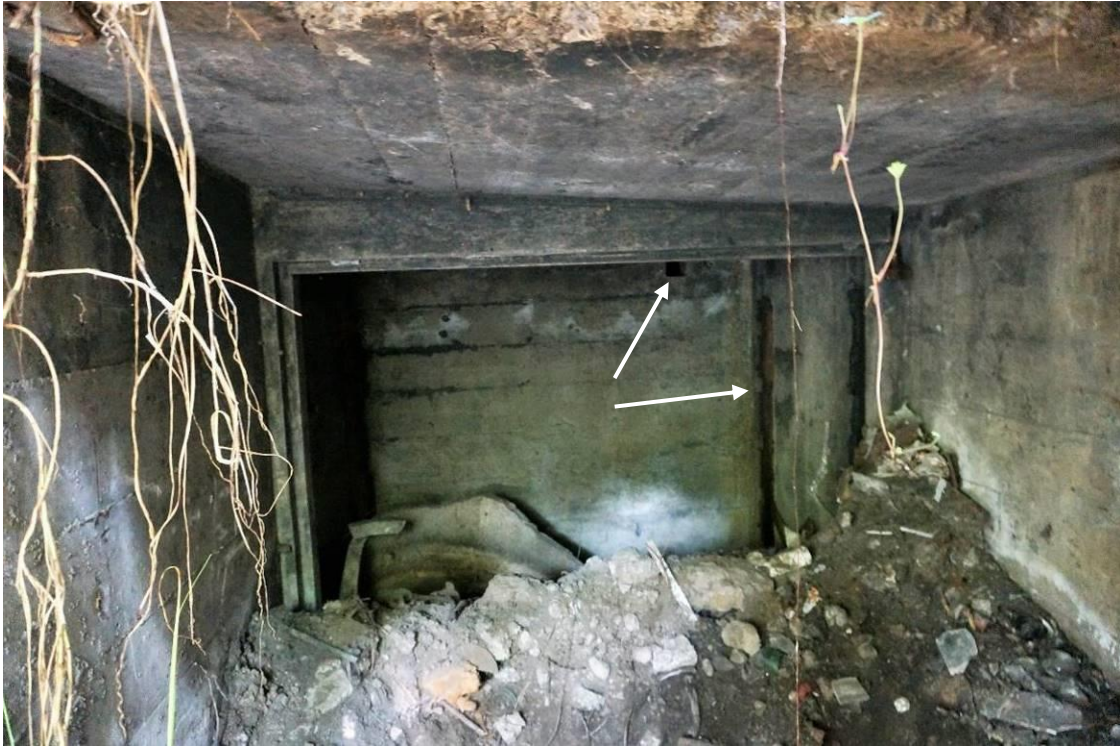
Figure 19. Southern emplacement, looking S towards southern ammunition recess. Note timber uprights for shelving and ventilation hole (arrows)
