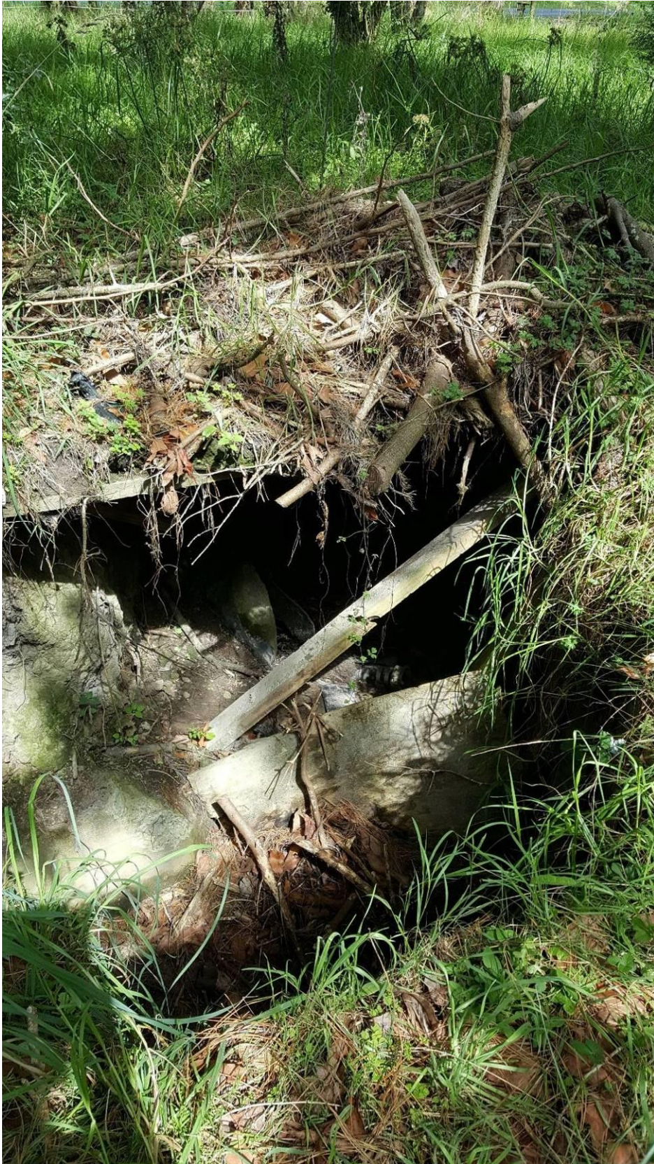
Figure 17. Southern emplacement looking S, showing collapsed timbers and soil/rubbish within the structure
