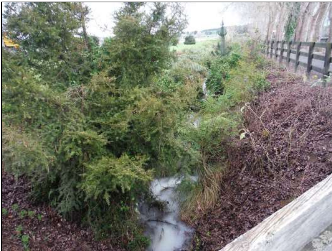
Figure 10 Main western drain as it runs in a straight channel beside the central driveway. Note the steep banks and discolouration of the water.
