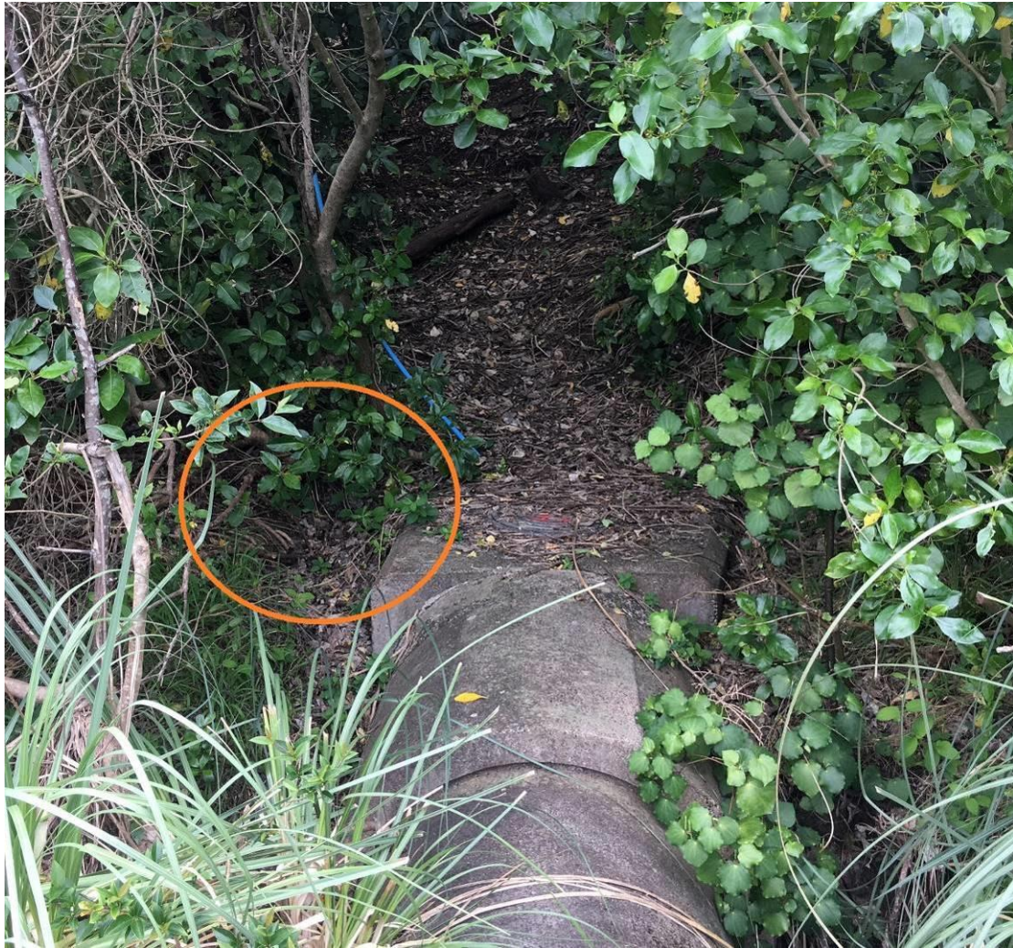
Figure 9 – existing WWMH1-0 with the proposed area of excavation ringed in orange. This is the termination point for the directional drilling
