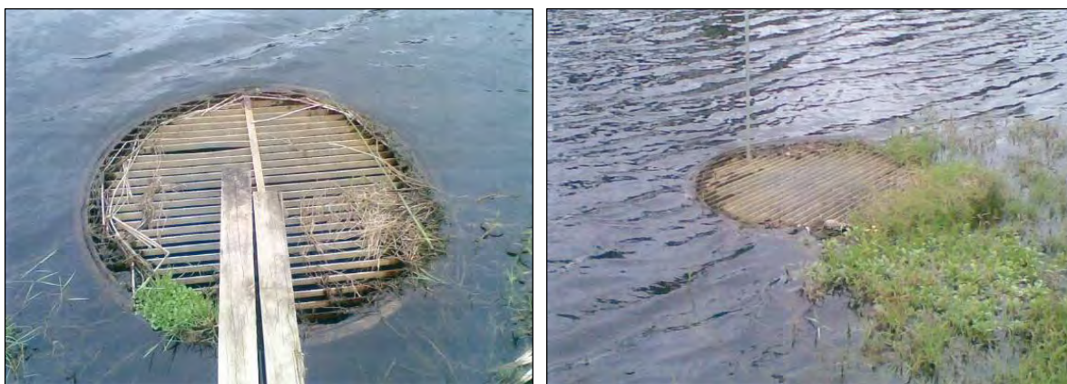
Figure 10: Pond 9 & 10 outlet structures.
